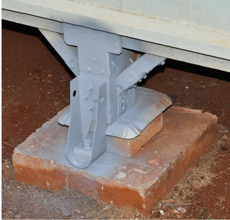
Figure 18: Galvanized connectors sprayed with zinc-rich cold-galvanizing paint to increase corrosion resistance. (To be followed by the second and third coats in the three-coat painting system)
